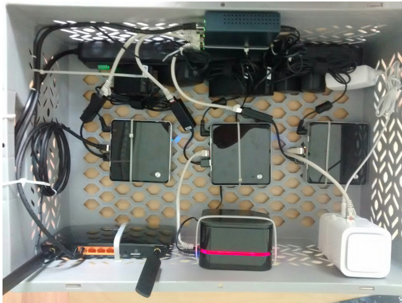
Figure 3.2: Installation of the used NUCs and LTE modems
